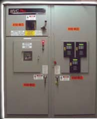
4160V, multi-motor Soft Starter designed to simultaneously start (3) 600HP conveyor motors.
